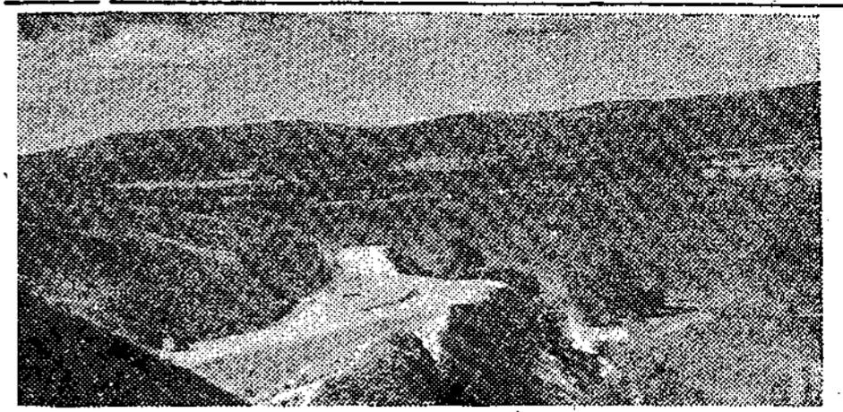
Cutting through the hills in the making of Highway 79 leading down to Okanagan Lake level was a big project as the picture illustrates.
