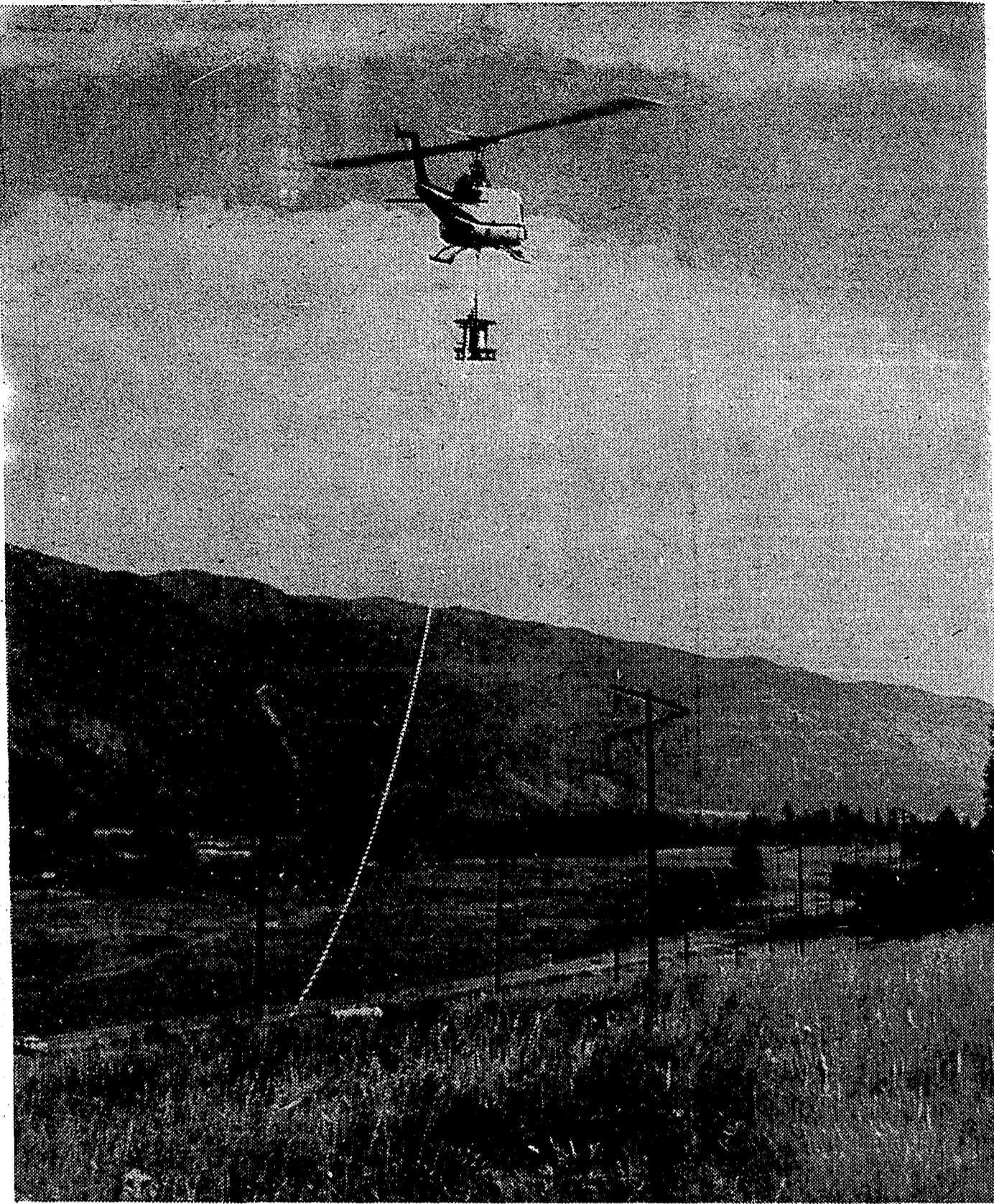
AN ESTIMATED 150 HOURS flying time was required to string conductor along a 38-mile-long right of way for a new 138,000-volt transmission line now nearing completion between Kamloops and Barriere. Pilot of this Okanagan Helicopters Ltd. aircraft with 3,200 pounds of conductor slung in a reel beneath the machine, is guided by men on ground with walkie-talkie radios. B. C. Hydro transmission line runs parallel to existing 60,000-volt line near the North Thompson River. Helicopter carries 6,000-feet of conductor on each lift.
