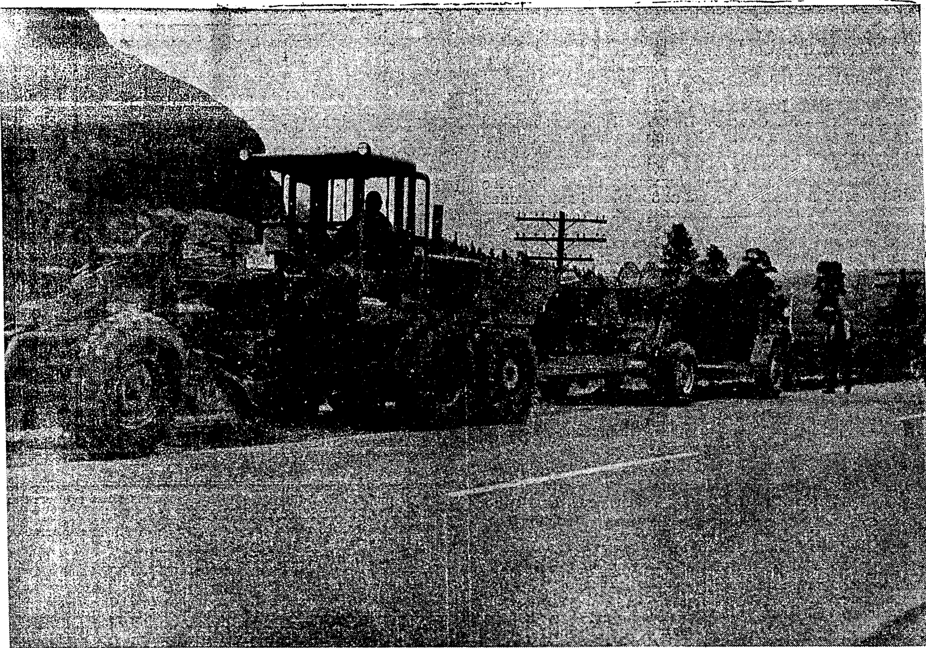
B.C. Telephone Construction crew ploughing cable underground in the Pritchard area between Kamloops and Chase.
